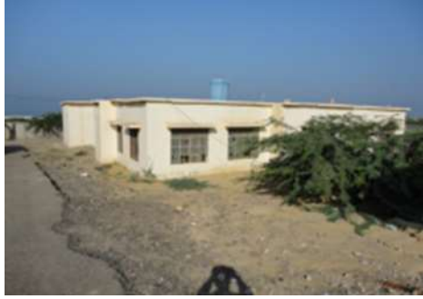
Hospital in the yard. The windows are broken.
